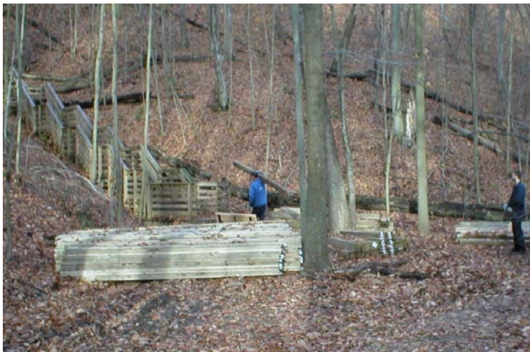
Here inmate workers haul treated lumber up the side of a hill, where they're constructing a stairway.
